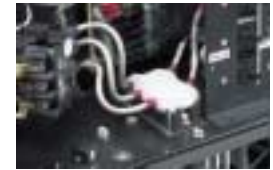
Coated Electrical Connections
